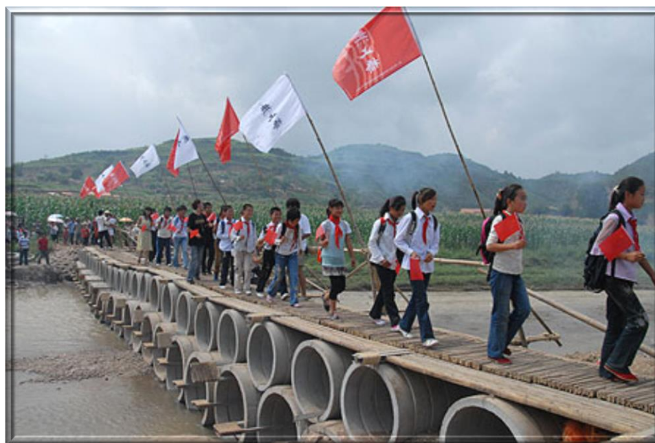
1 August 2009 -- This 27M long “Tàibái Wú Zhǐ Qiáo” (太白無止橋) in Gansu Province (甘肅省) was the joint project by students from The Chinese University of Hong Kong (香港中文大學), The Hong Kong Polytechnic University (香港理工大學), and Xi'an University of Architecture and Technology (西安建築科技大學).
